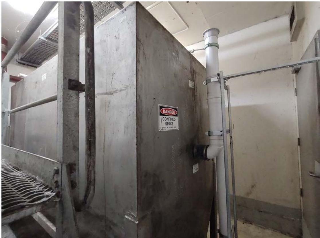
Photo 20: Grease arrestor room in basement 2
