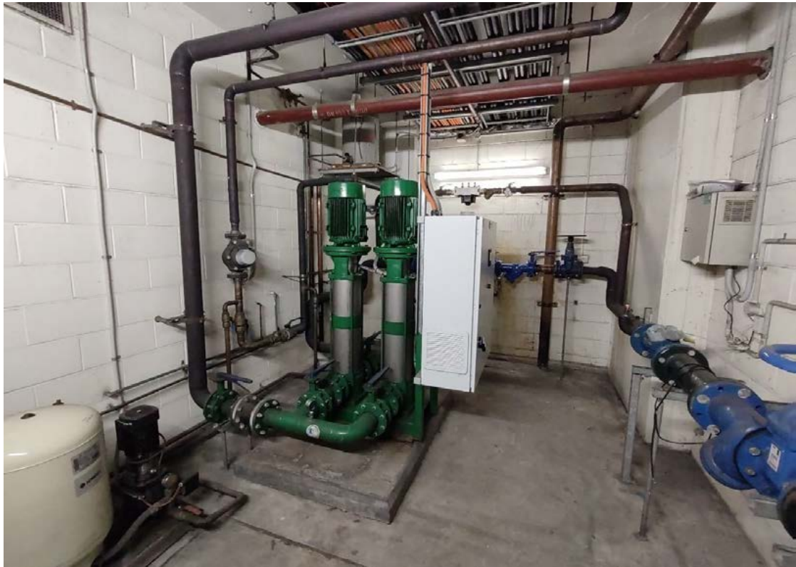
Photo 19: Water pump room in basement 2
