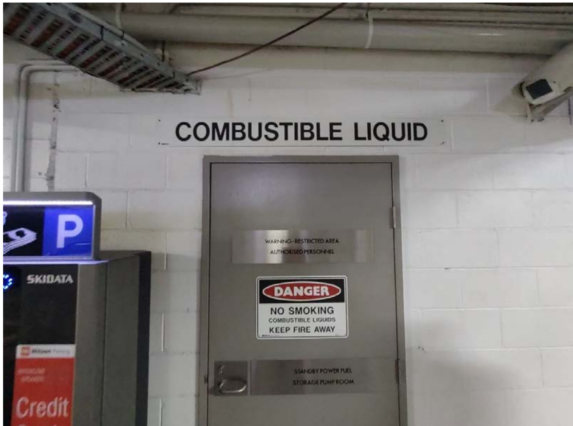
Photo 4: Standby power fuel storage pump room
