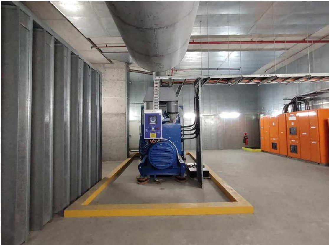
Photo 12: Diesel generator room in level 7
