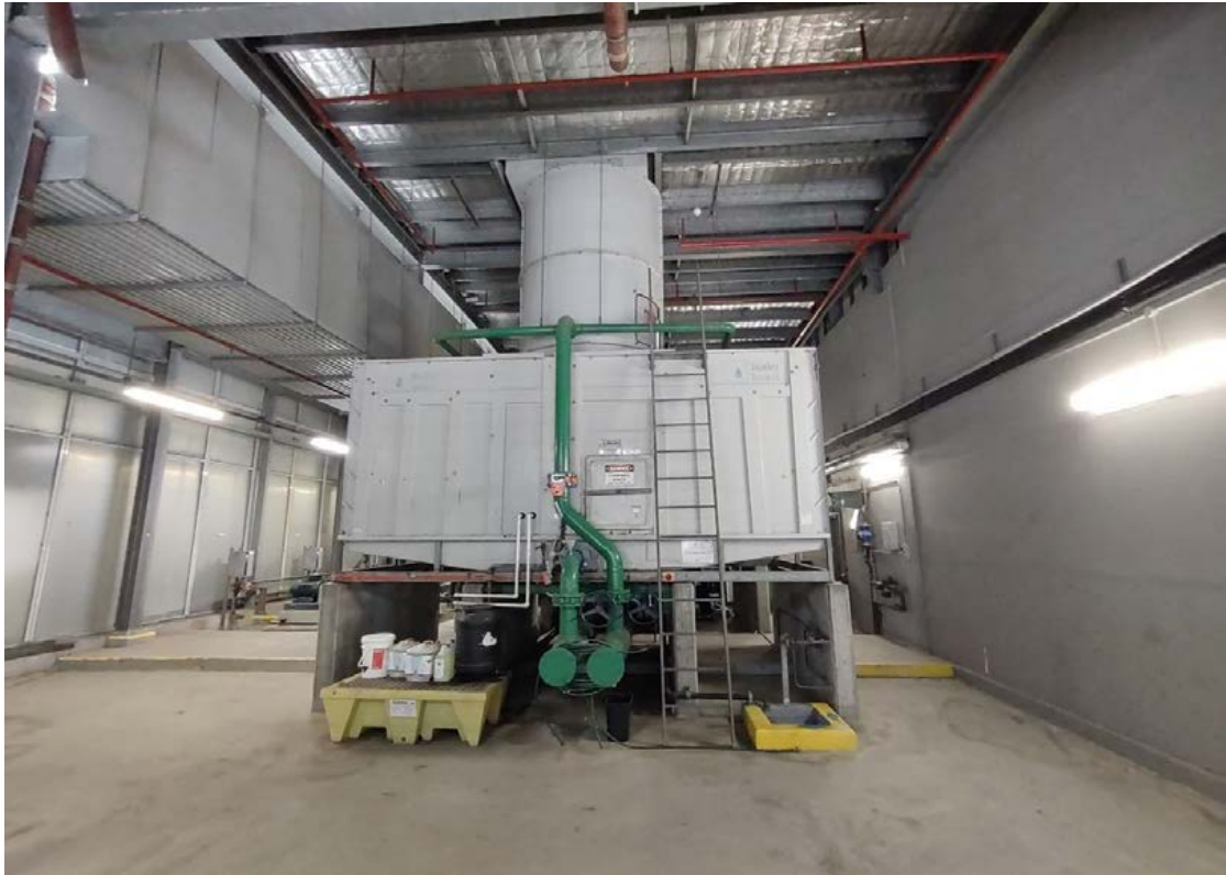
Photo 5: Coolin tower room in level 19
