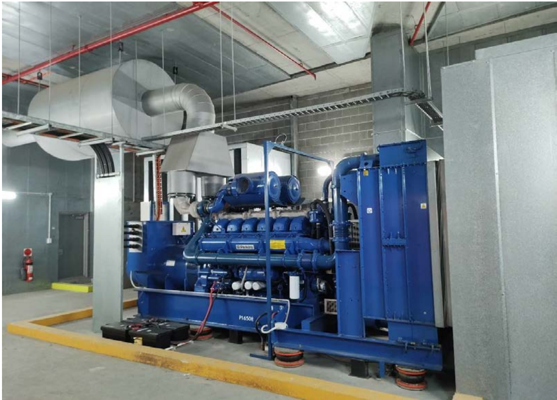
Photo 11: Diesel generator room in level 7
